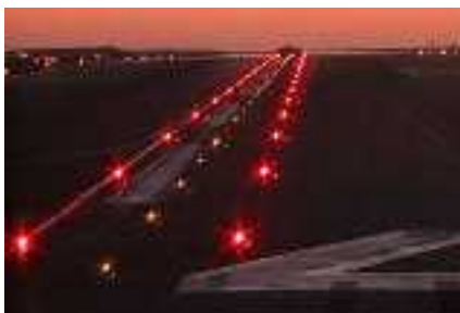
Figure 1: Runway Safety Lights.
